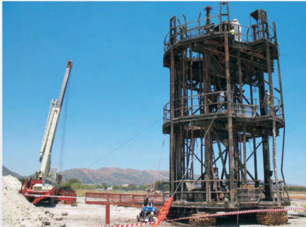
The stage being placed on wooden blocks by means of a 450 tonne crane
